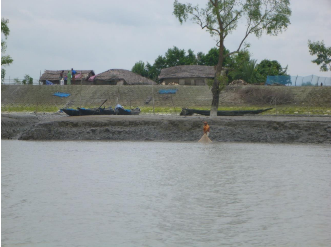
Figure 1. . Pictures showing embankments on Polder 32 from the embankment (top) and from the tidal channel (bottom).
