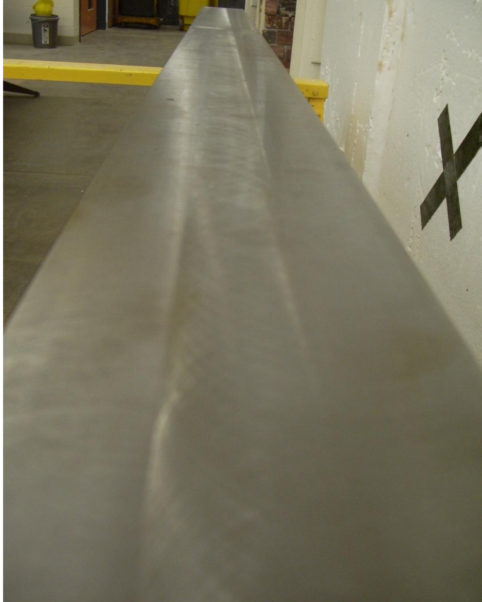
Figure 31. Close up view of bottom flange of beam SBI
