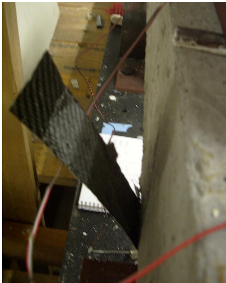
Figure 159. LTC 4300 debonding from concrete substrate
