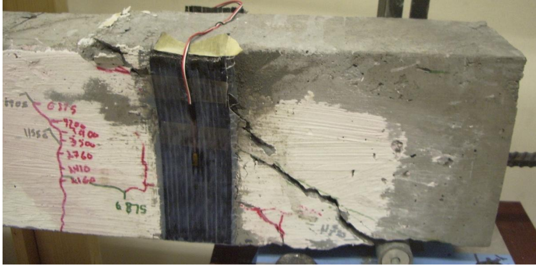
Figure 155. Shear crack in test beam 4
