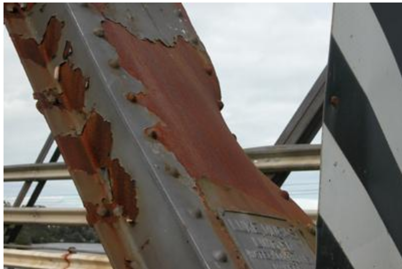
Figure 2. Corrosion of diagonal steel brace in addition to impact damage
