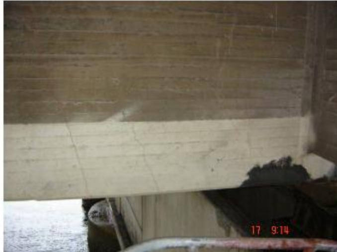
Figure 6. Diagonal shear cracks near support
