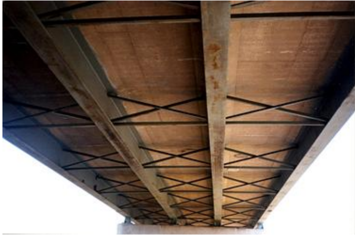
Figure 1. Corroded girder of Chesterfield Bridge in Virginia
