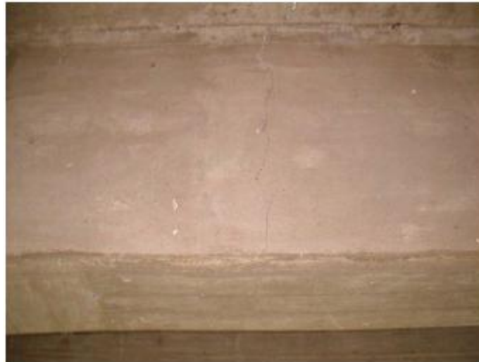
Figure 4. Reinforced concrete beam with vertical crack
