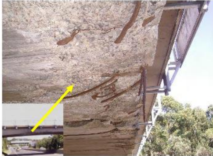
Figure 6. Overhead vehicle impact damage to bottom of prestressed girder
