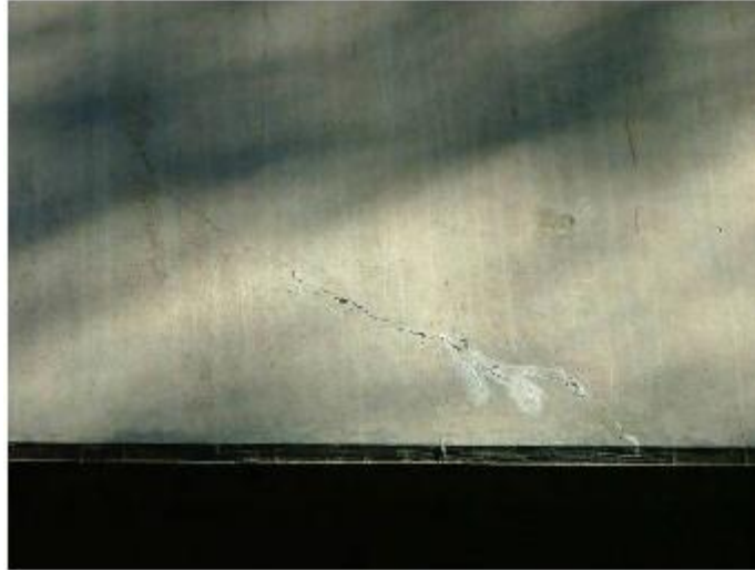
Figure 8. Diagonal crack in prestressed girder
