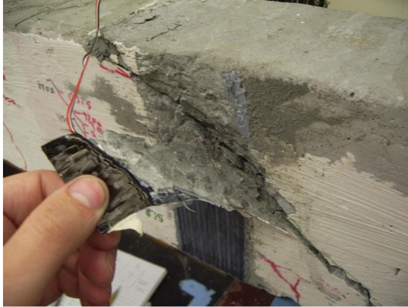
Figure 157. Close up of concrete cover separation of test beam 4
