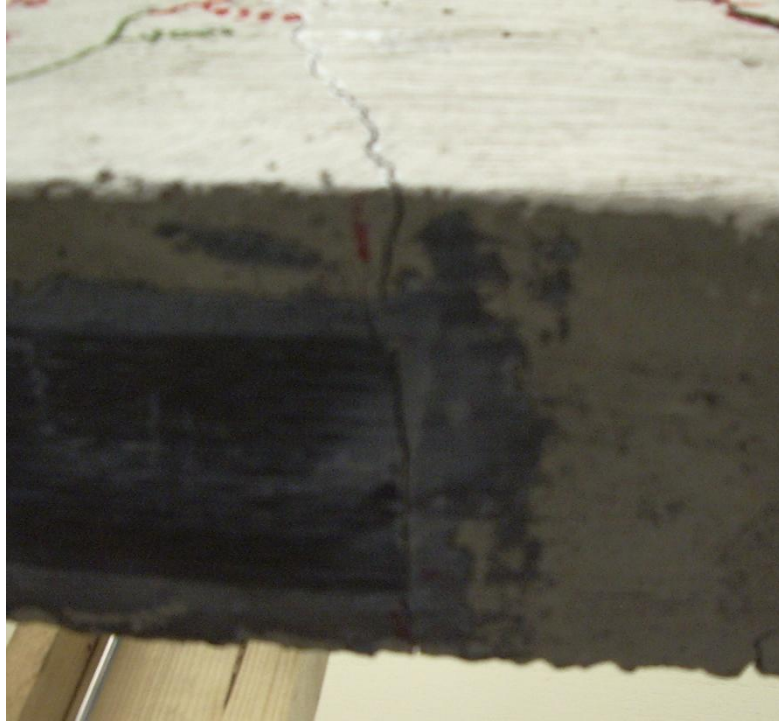
Figure 150. Crack development in the bottom of beam at Sikawrap edge
