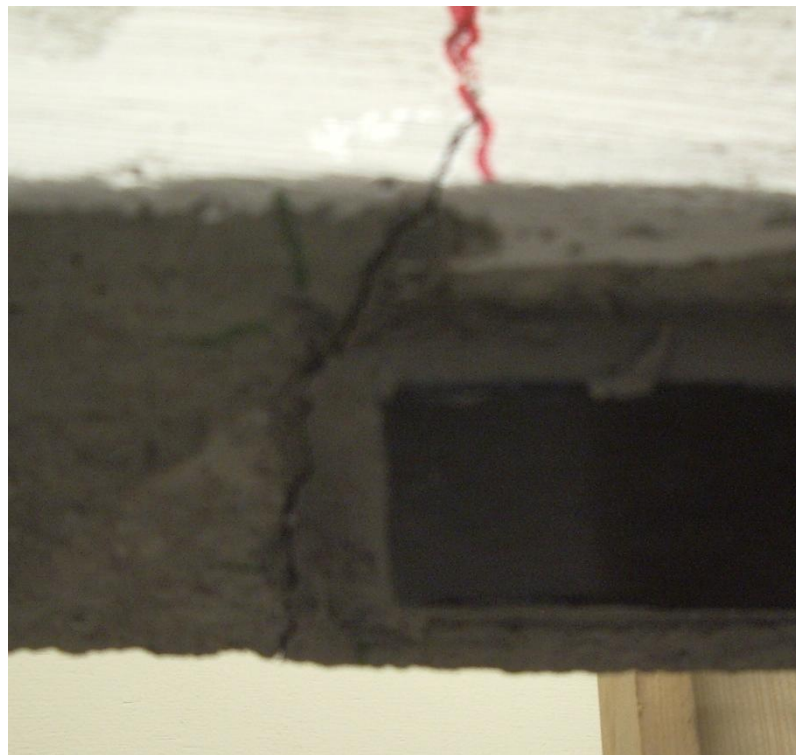
Figure 151, Crack development at the patch edge of a Carbodur patch
