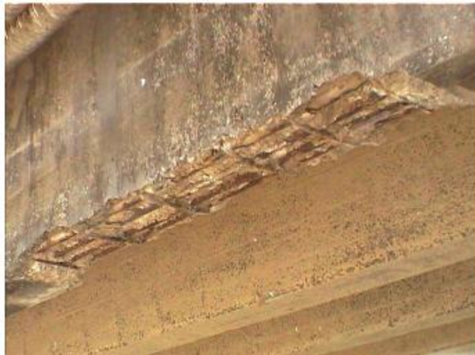
Figure 5. Severe spalling and delamination, exposing corroded reinforcing steel
