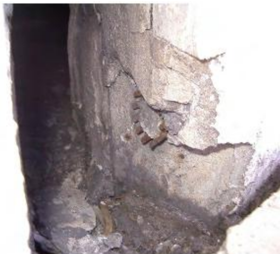
Figure 7. Deterioration of prestressed girder end, exposing anchorage
