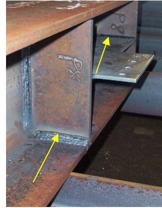
Figure 8: (Steps 6-9 and 10-13) Turn the column onto its flange and weld at the above locations and other similar locations
