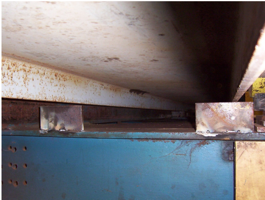
Figure 35: The beam lifting off its support due to lateral-torsional buckling
