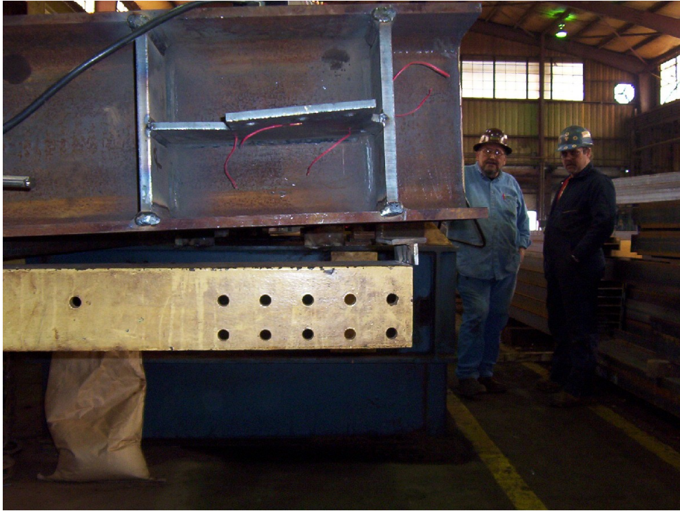
Figure 34: The column lifting off its support due to lateral-torsional buckling of the beam
