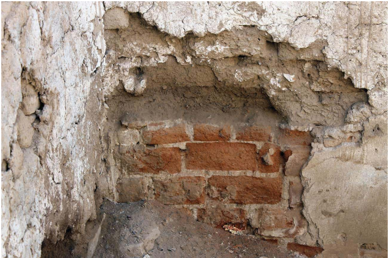
Figure 7.9. Detail of colonial brick and lime foundation of the structure adjacent to the east of the chapel at San Pablo.
