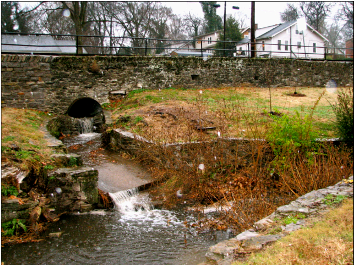
Figure 5. This metal culvert feeds into the stream into Sevier Park, carrying stormwater from beneath the streets of Nashville into the body of water. (photo by Jennifer Mokos)
