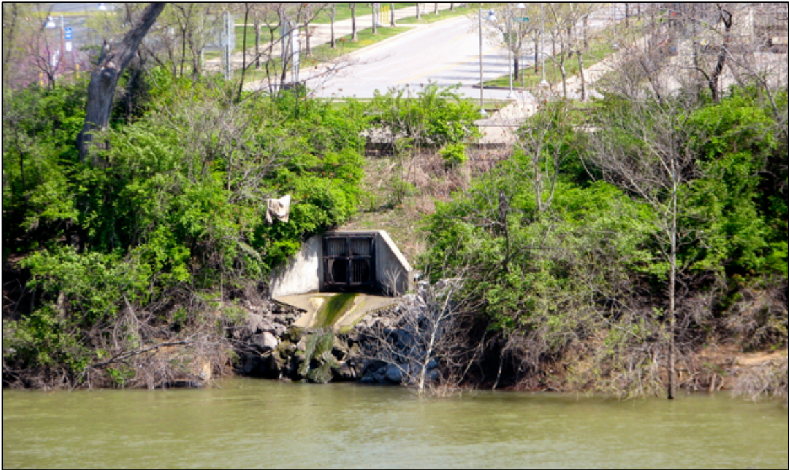
Figure 31. Outflow pipe on the east bank of the Cumberland River near the LP Field football stadium (photo by Jennifer Mokus)
