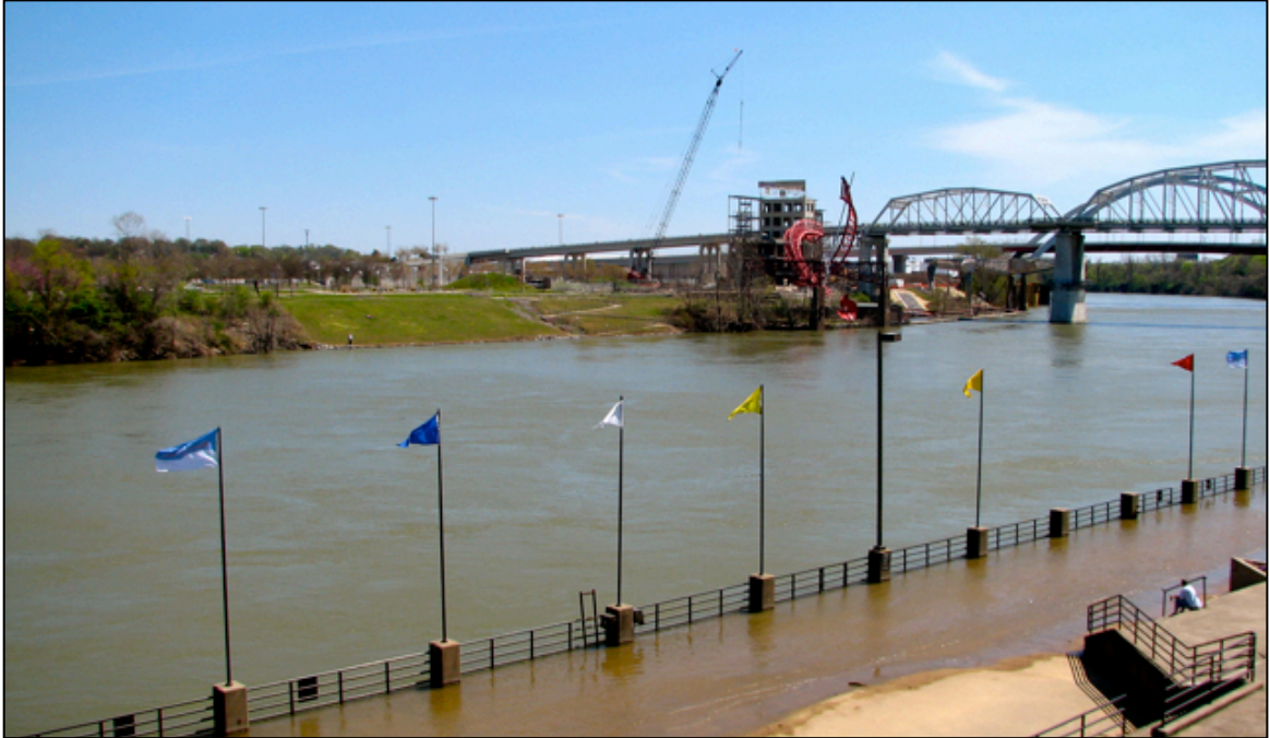
Figure 30. A water play park and office building under construction on the east bank of the Cumberland River across from Riverfront Park. (photo by Jennifer Mokus)
