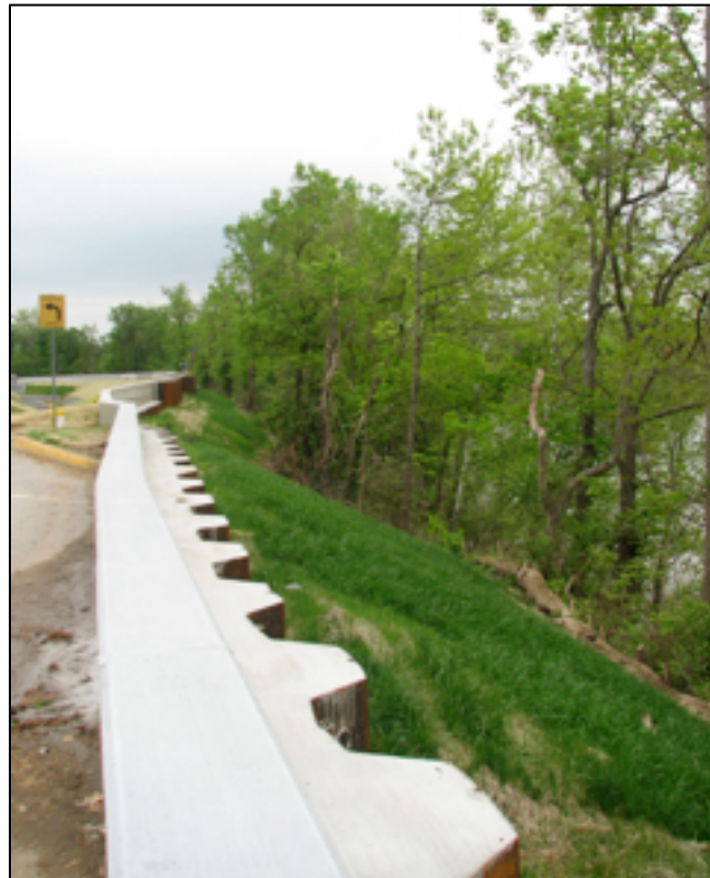
Figure 34. The Opryland levee following repairs to the damage caused by the 2010 flood. (photo by Jennifer Mokos)
