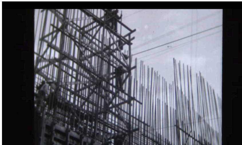
Figure 1.8 A shot of the Grand Coulee Dam's cathedral-like rebar structures in Hydro
