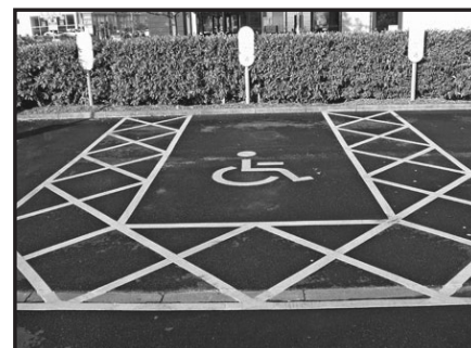
The new, better handicapped spots are fit for a disabled king.
