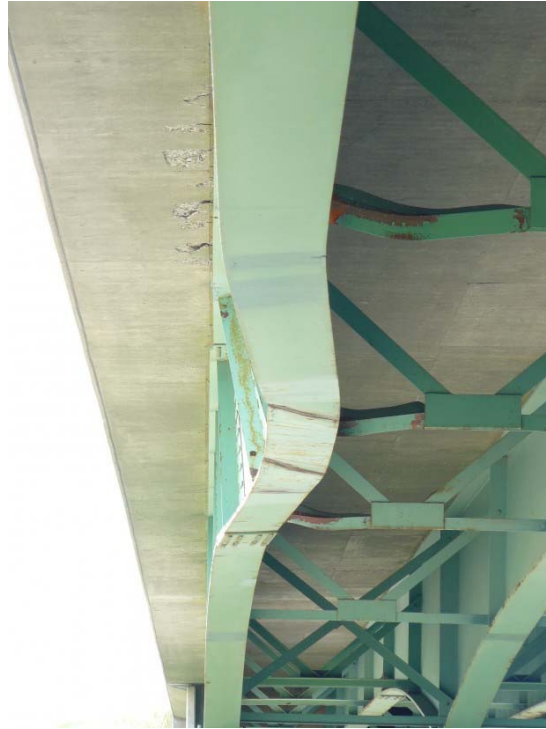
Figure 1.2.12. Bent steel girder due to impact damage.
