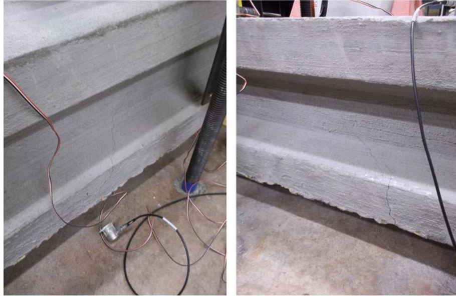
(a) Detached sensor (Channel-1) at first crack location
