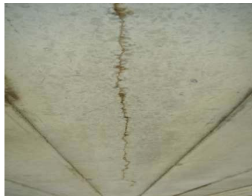
(b) Longitudinal crack
