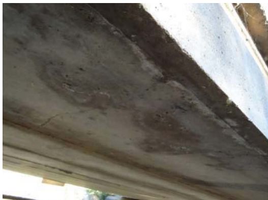
(a) Flexural cracks
