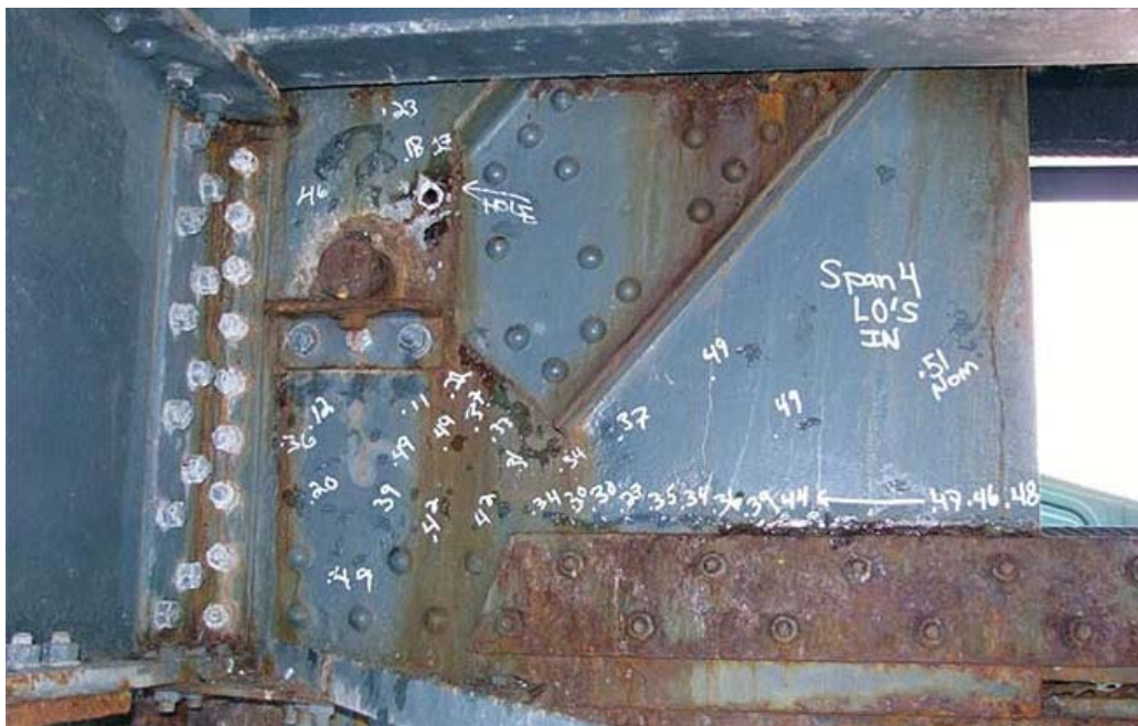
Figure 1.2.11. Corroded plates of Stillwater Bridge in Minnesota.
