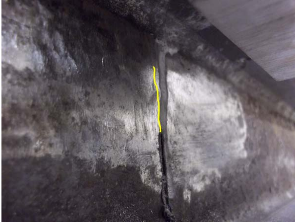
Figure 2.2.15. Crack formation in steel beam SB-1 (highlighted).
