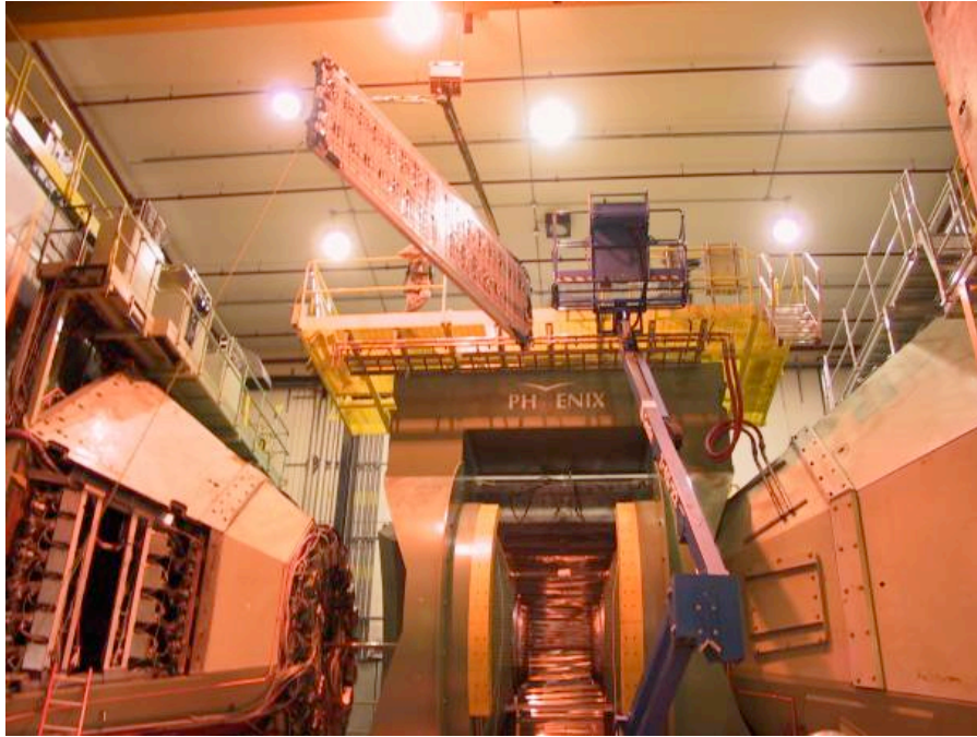
FIGURE A.1. TOFW Sector Installation (PHENIX IR)
